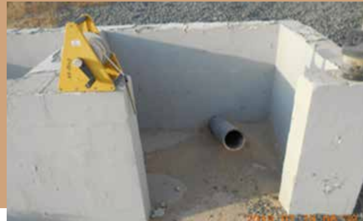
Figure 38. Leachate Inspection Pipe in the landfill.
