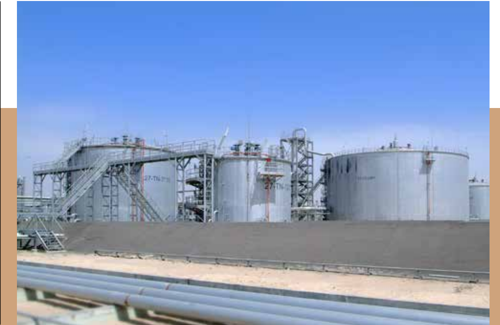
Figure 22. Recovered oil in storage tank.
