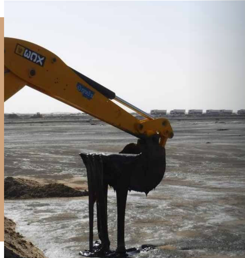
Figure 24. Wet oil lake before remediation (2016)
